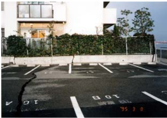
Figure 4. Photograph showing cracking at parking lot and fence parapet on the west side.
