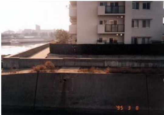
Figure 5. Photograph showing cracking on the quay wall to the east of the building.
