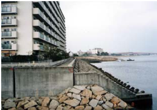
Figure 2. Photograph showing closer view of the south-west corner, where the widened gap due to bulging out of the quay wall towards the sea can be clearly seen.
