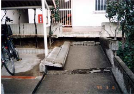
Figure 6. Photograph as seen from the north side of block A, where gap developed under the corridor and the crack parallel to the building about 5m in front may be noticed.
